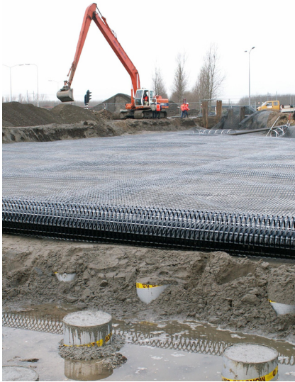
Figure 2. Weak soil conditions
