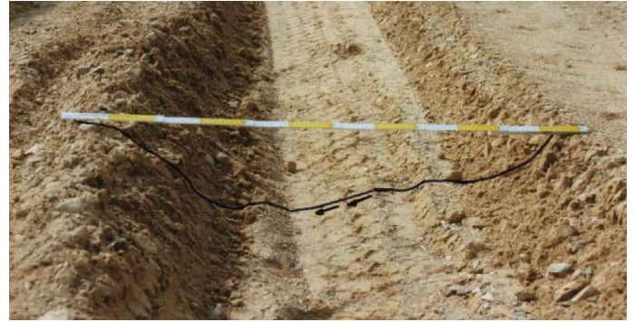
Figure 3: Rutting on a construction site
